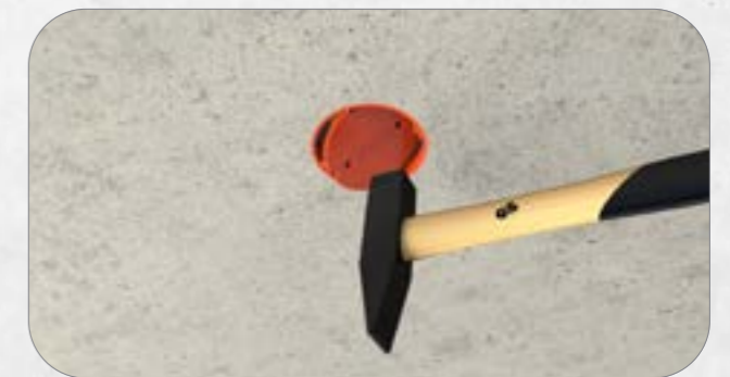
4. Close the box with the cover and concrete the ceiling. Tap in the Front part with a hammer after concreting.
